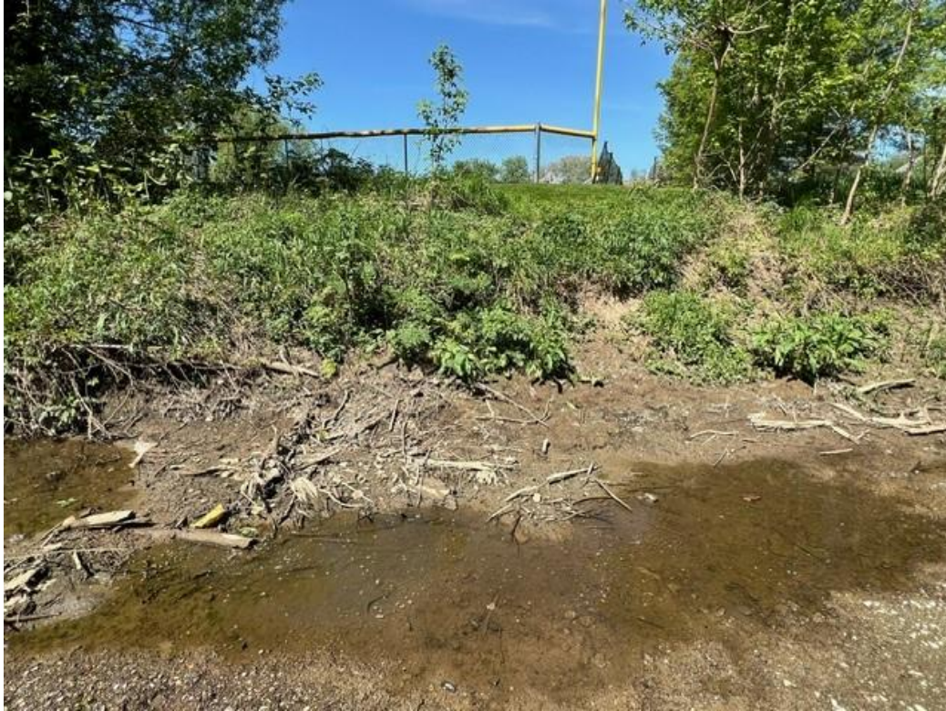
Figure 8. Erosion at subsection C, shown on May 3 rd , 2024.
