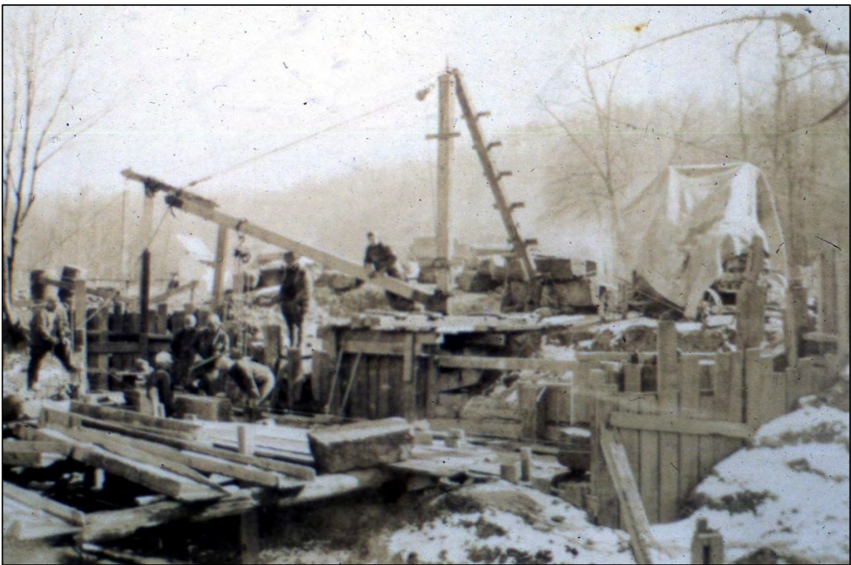
Figure 2.5: Civilian Conservation Corps workers use a pulley-rigged crane to help build the dam at the upper lake, ca. 1935. Notice the light covering of snow on the job site. Photo courtesy of Raccoon Creek State Park Archives.
