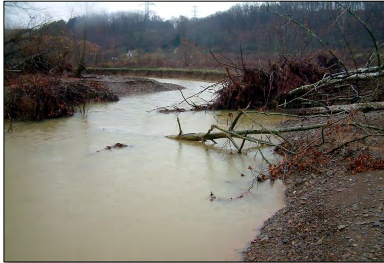
Figure 4.5: Flood damage on Raccoon Creek at Independence Marsh. 11/4/2004.
