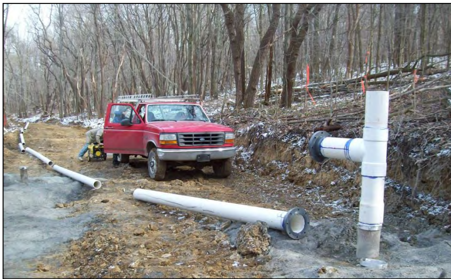
Figure 4.23: A crew from BioMost, Inc. installs temporary piping to conduct a flow test from Raccoon Creek to Erie Mine, part of the feasibility study for the "ELF," the proposed treatment system for Erie, Langeloth and Francis Mines in Burgettstown, 2/4/2010. Photo courtesy of BioMost, Inc.
